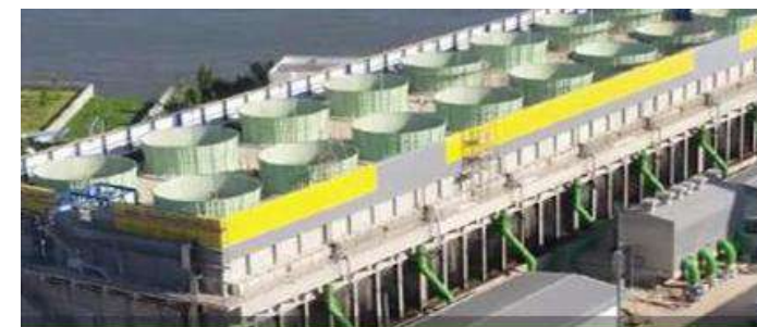
Mechanical Draft Cooling Tower (cellular)
